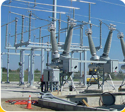
EHV SUBSTATION & DISTRIBUTION
